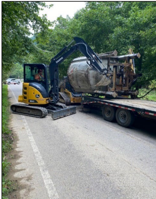
Photo 13: Southeast KY Flooding – Spill Response
